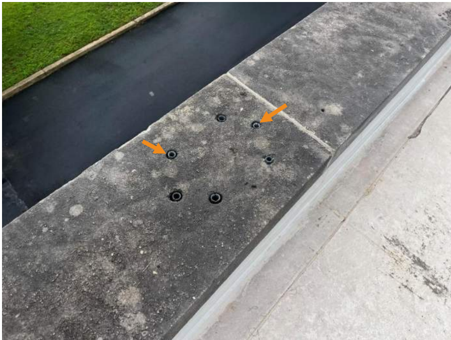
Figure 66. Abandoned anchors in the coping.
