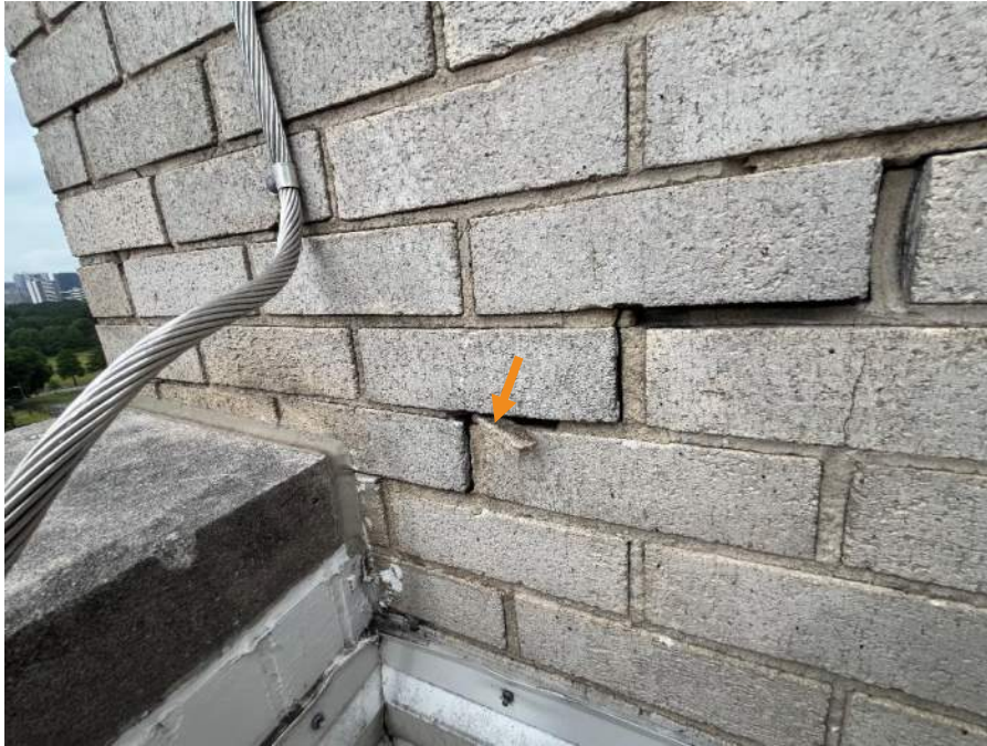
Figure 25. Areas of loose or missing mortar along stair-stepped cracking at mechanical penthouse.
