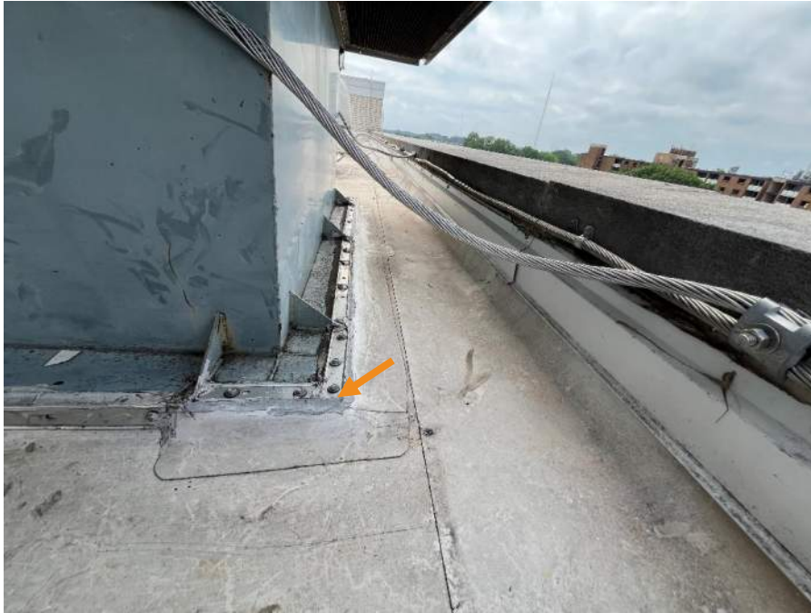
Figure 107. Low curb height on mechanical penthouse roof
