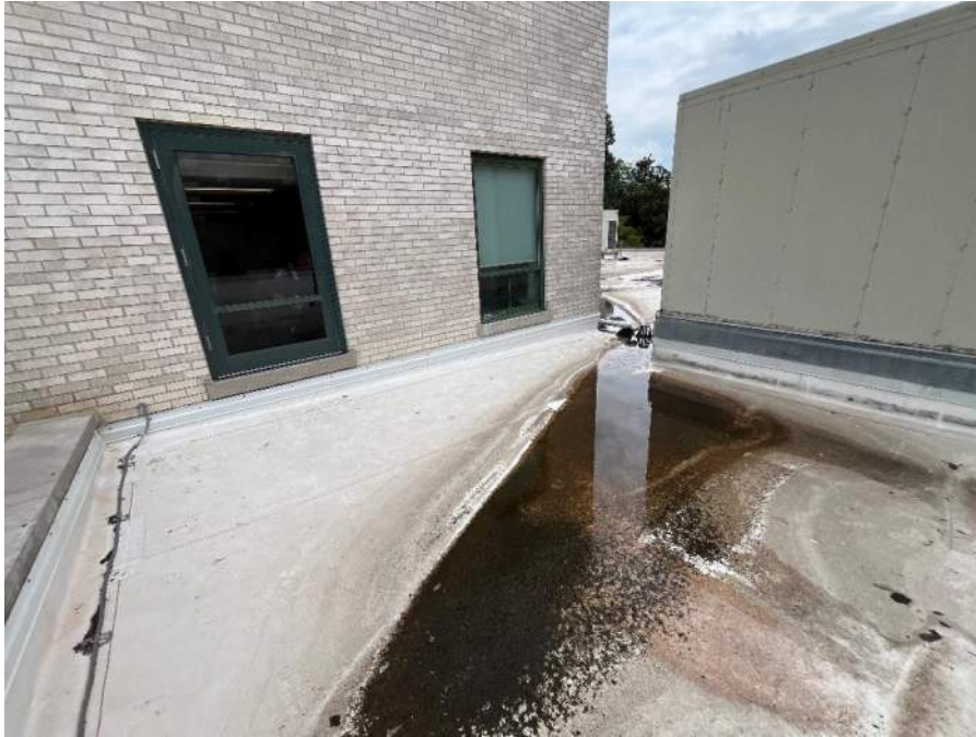
Figure 97. Ponding water at the western half of the main roof and east low roof was concentrated around obstructed roof drains
