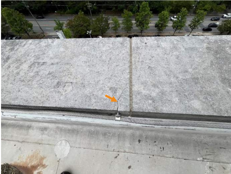
Figure 67. Cracking in the coping at lighting protection anchors.
