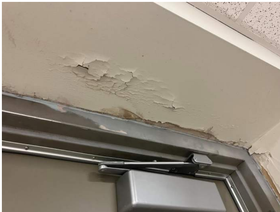
Figure 12. Close-up view of peeling and stained finishes in Figure 11.
