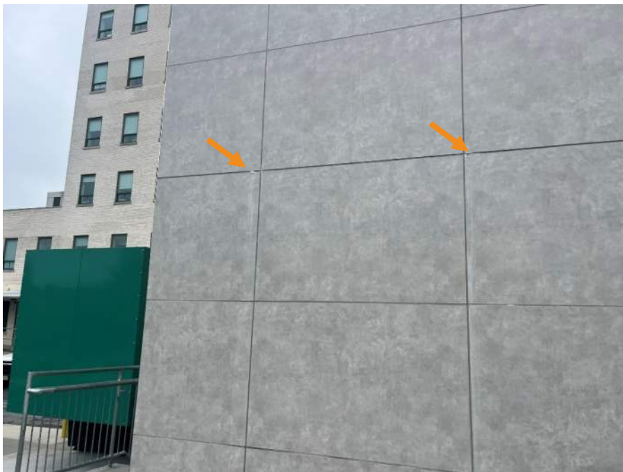
Figure 80. White staining emanating from the sealant bed joint on the west side of the main entrance.
