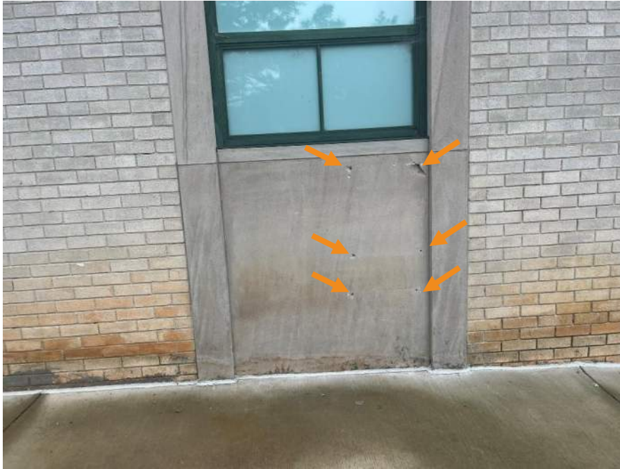
Figure 65. Six abandoned anchors at one wall panel at grade on the north facade.
