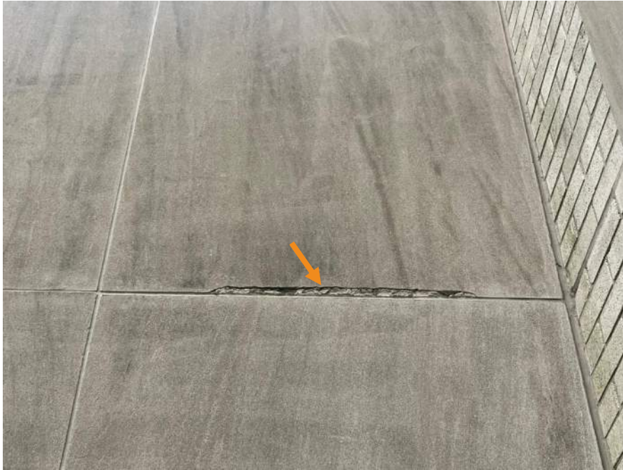
Figure 49. Spalling along panel edge.
