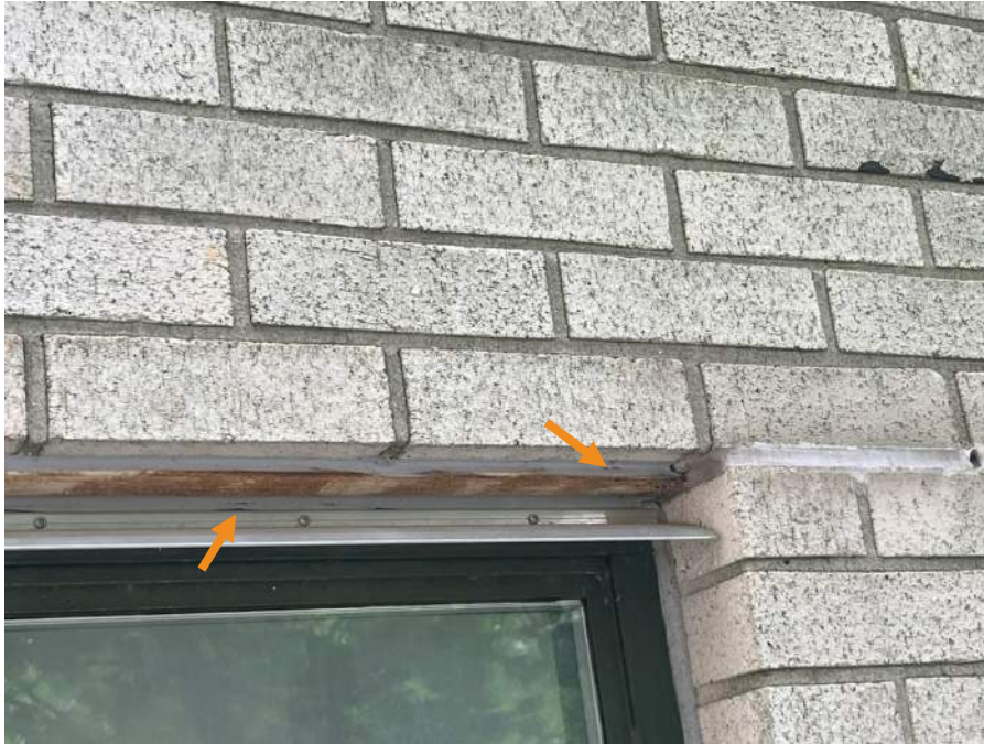
Figure 87. Adhesive and cohesive failures of sealant at a courtyard window.
