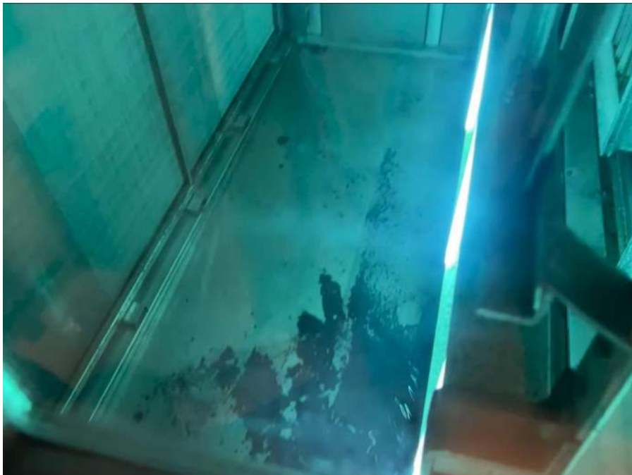
Figure 110. Inaccessible area of mechanical system with standing water at floor
