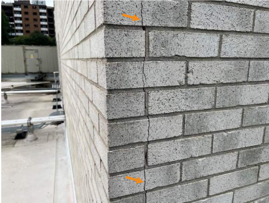
Figure 23. Vertical cracking at the northeast building corner viewed from the low roof.
