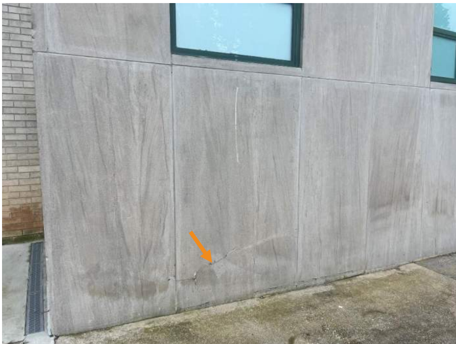
Figure 48. Cracking at north facade panel at grade adjacent to the north drive aisle.
