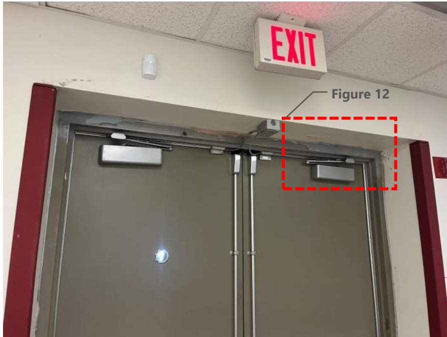
Figure 11. Peeling finishes and staining at ambulance bay entrance.
