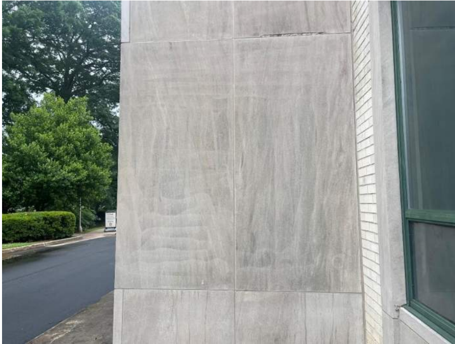
Figure 55. Uneven panel discoloration at panels accessible from grade.
