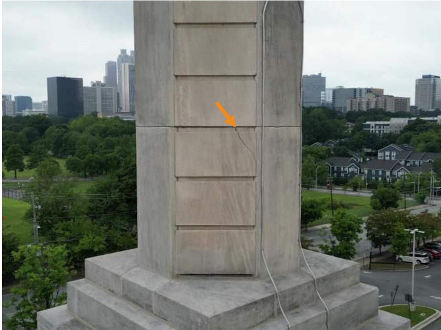
Figure 51. Cracking at south facade steeple panel.
