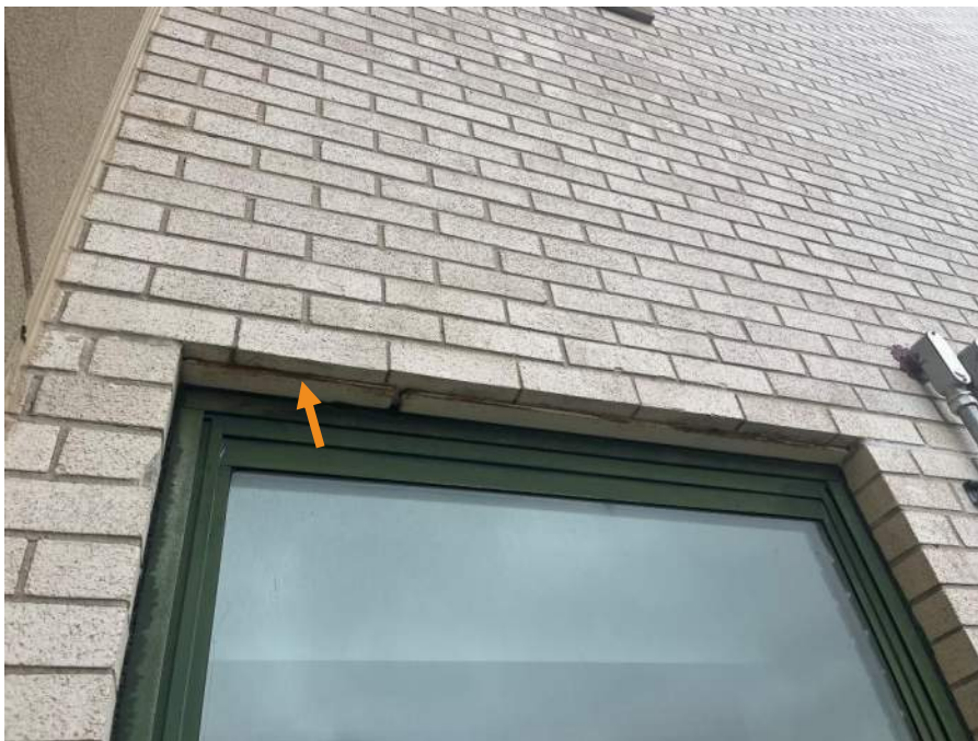
Figure 36. Light surface corrosion on visible surface of steel angles spanning over window.
