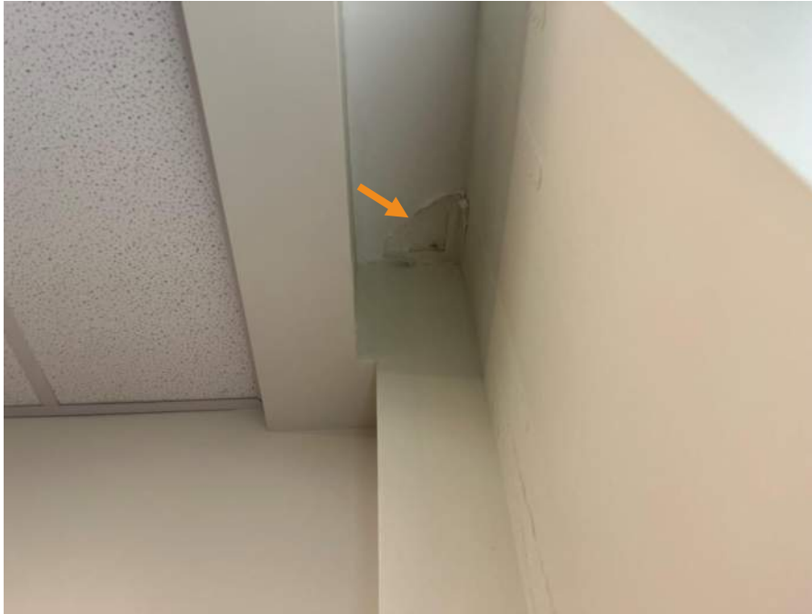
Figure 9. Interior finish coating peeling at northwest corner of Office 6022.
