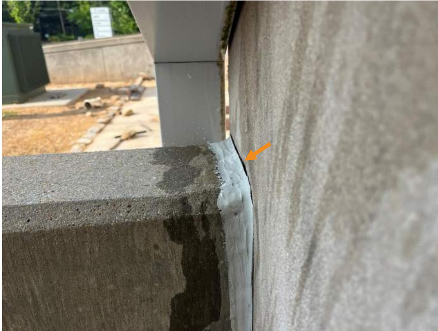
Figure 63. New sealant adhesively failed between the concrete knee wall and limestone panels.
