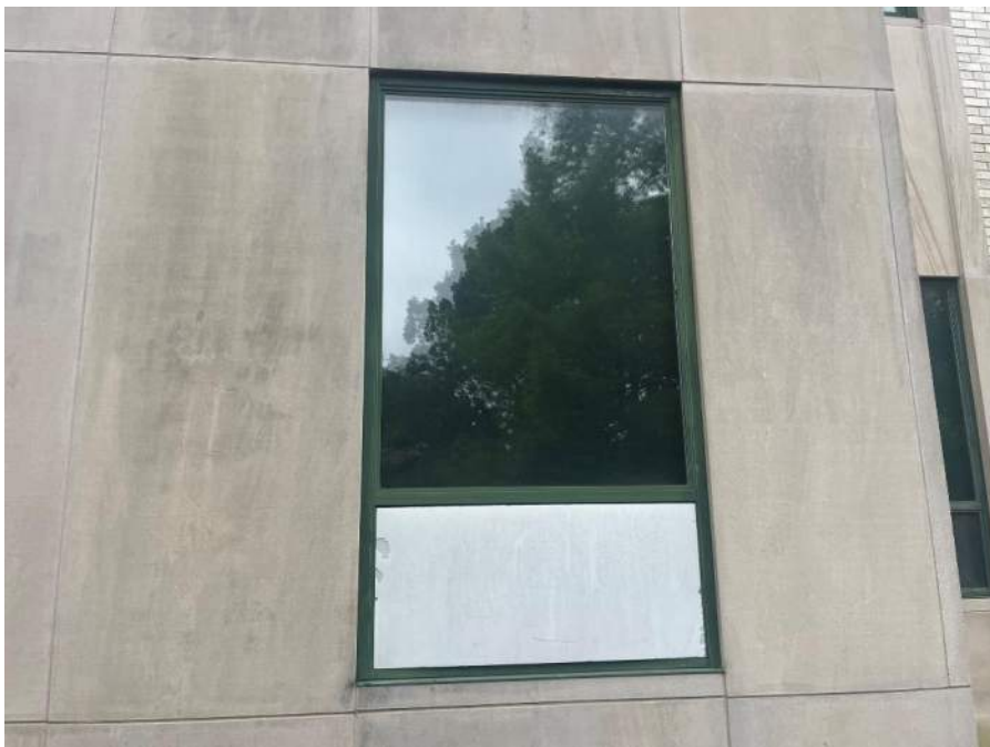
Figure 90. A foam panel covered a broken lite on the north side of the east wing
