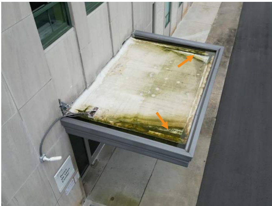
Figure 98. Ponding water on the north entrance canopy.
