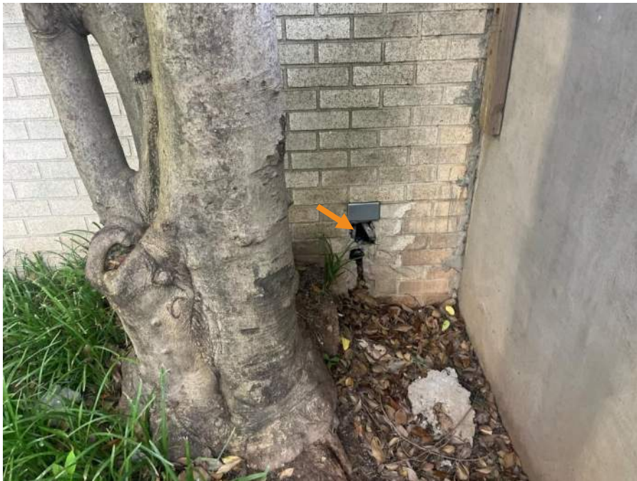
Figure 38. Missing brick units.
