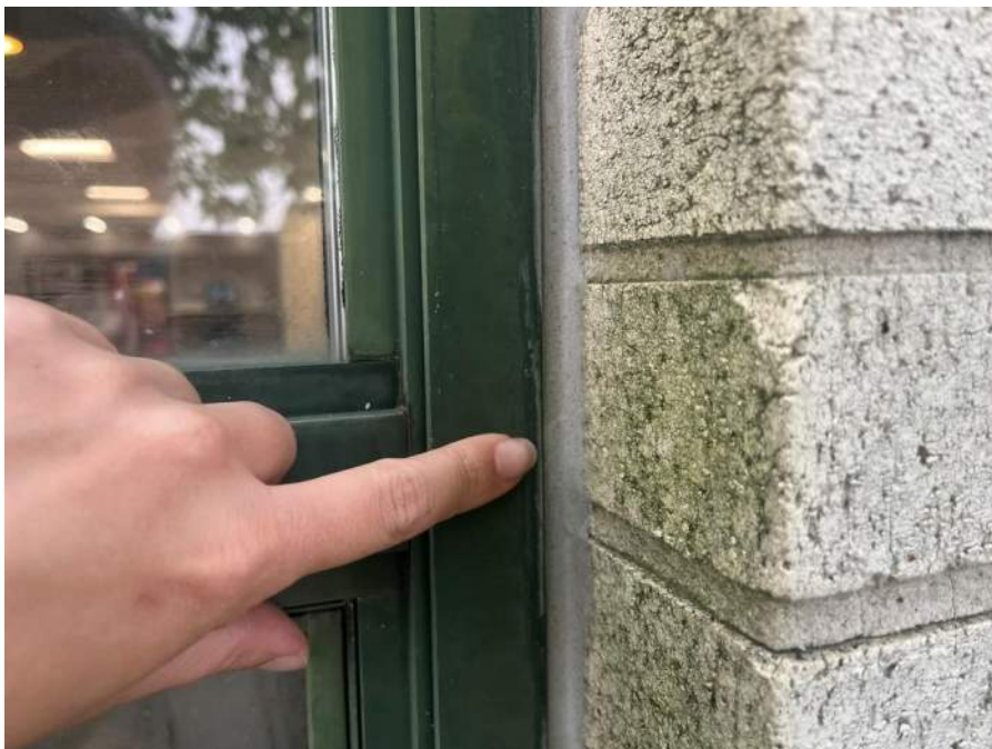
Figure 84. Gray-colored window perimeter sealant in the courtyard.
