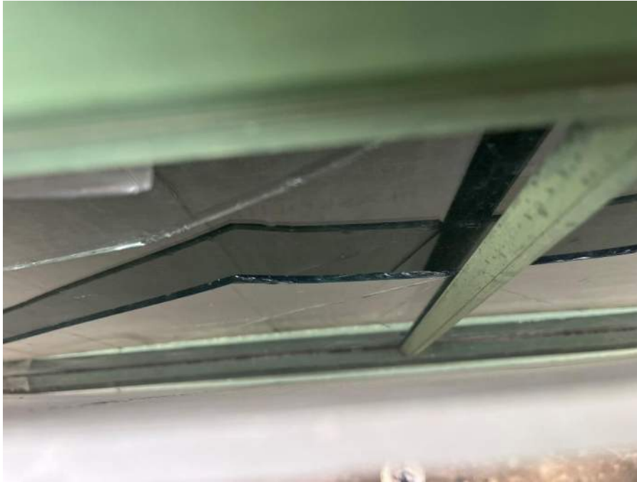
Figure 91. Broken lite on the north side of the east wing.
