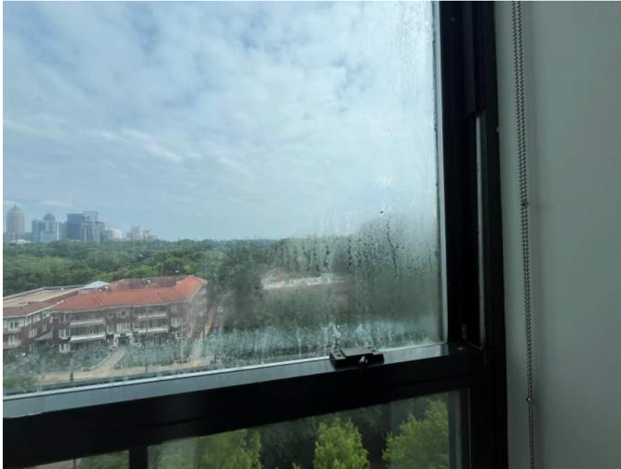
Figure 17. Fogged IGU at window assembly.
