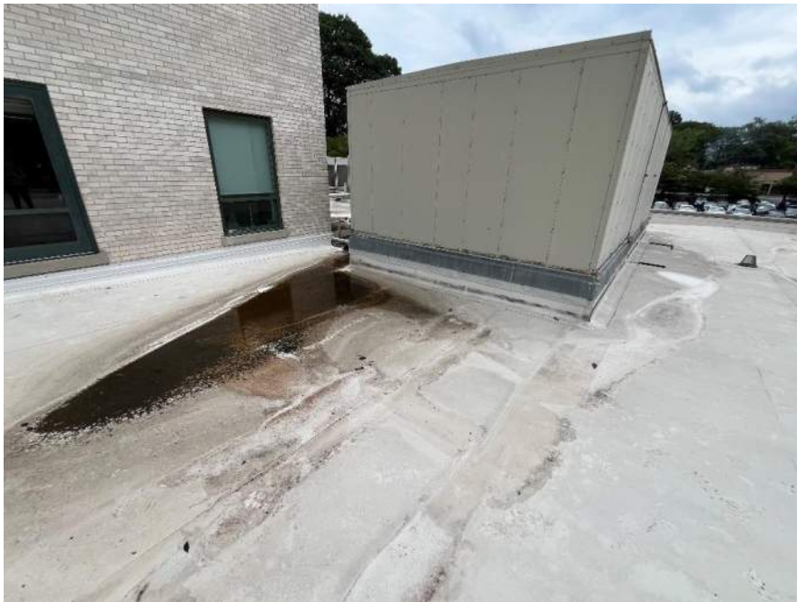
Figure 108. Overview of mechanical system at east wing low roof, located above stained ceiling tiles observed at Level 1 ceiling
