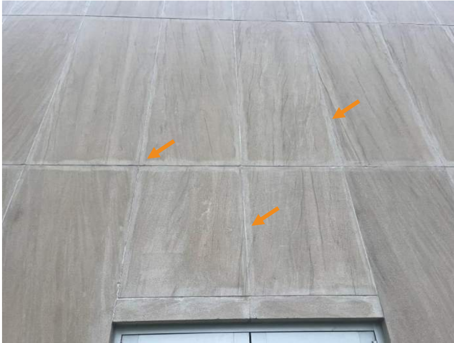
Figure 53. No staining present approximately 1 to 2 inches from panel joints.
