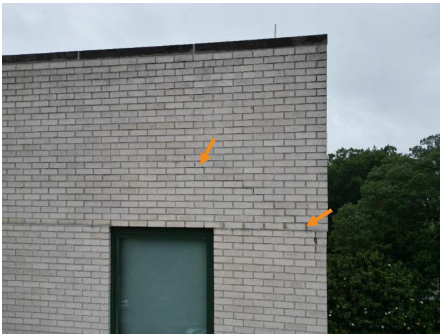
Figure 24. Stair-stepped mortar joint cracking at the main roof southeast building corner.
