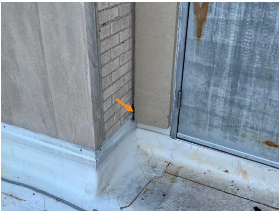
Figure 76. Missing sealant at the joint between the EIFS and adjacent brick return at the west facade.
