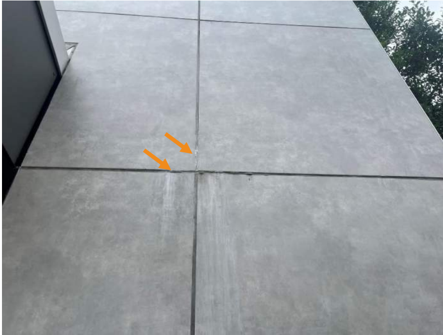
Figure 79. White staining emanating from the sealant bed joint on the east side of the main entrance.
