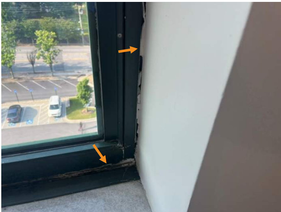
Figure 6. Stained and separated finishes at stairwell window.
