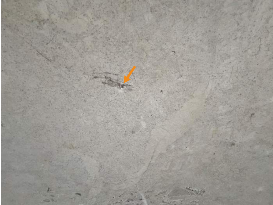
Figure 99. Punches and scratches on the roof membrane
