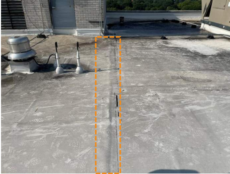
Figure 101. Isolated blisters at the membrane lap
