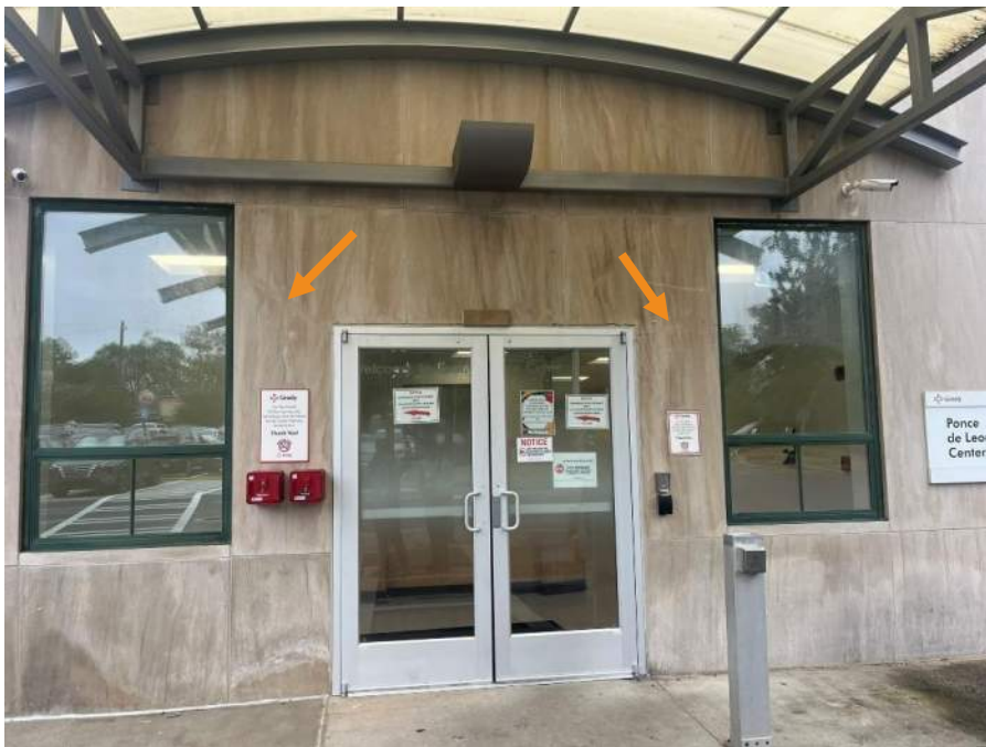
Figure 46. Cracking in L-shaped panels at east wing employee entrance head-to-jamb reentrant corners.
