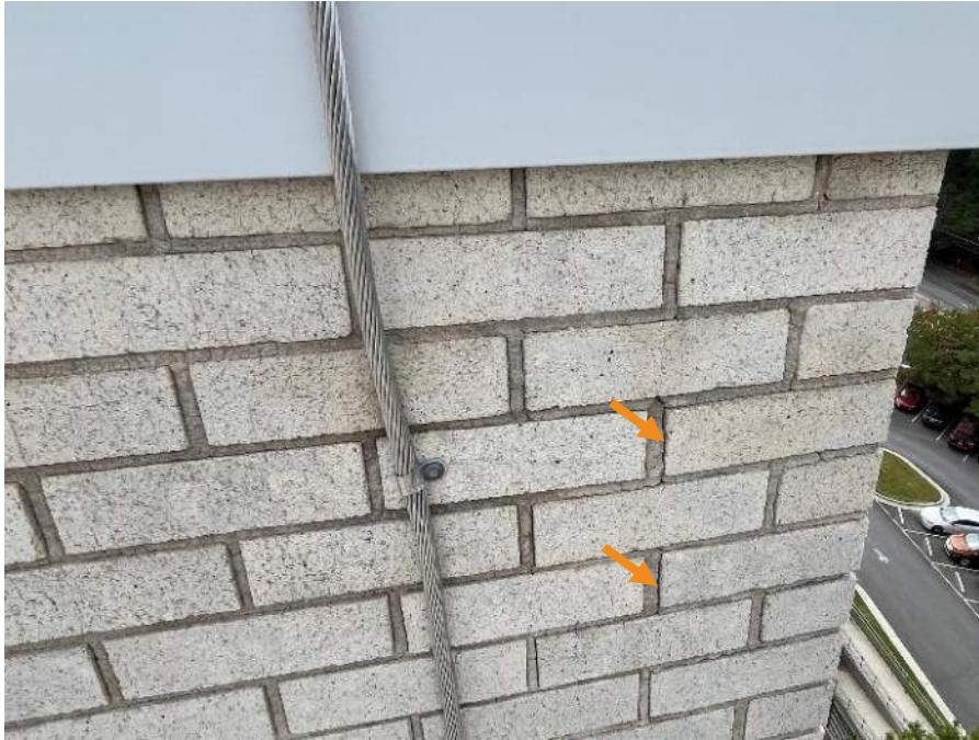
Figure 27. Area of mortar joint bond separation.
