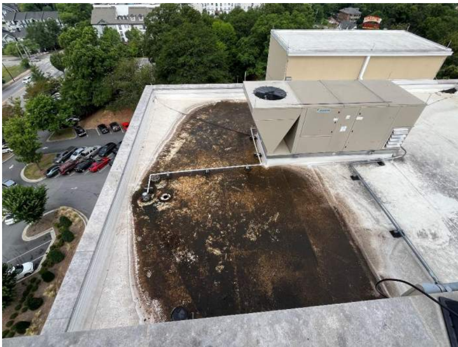
Figure 96. Ponding water at the western half of the main roof and east low roof was concentrated around obstructed roof drains
