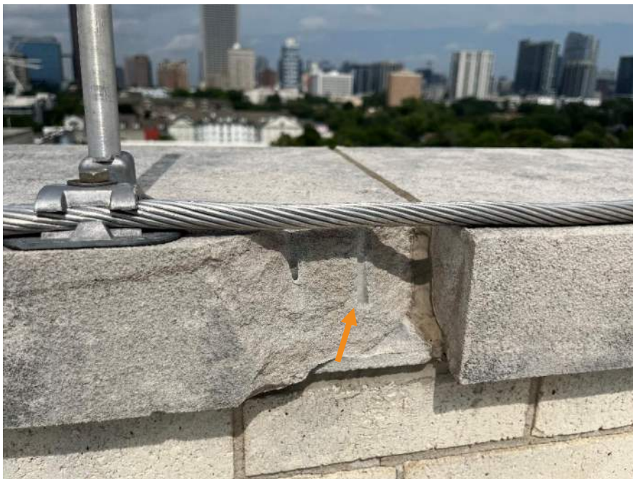
Figure 68. Spalls in the coping at previously installed anchors.
