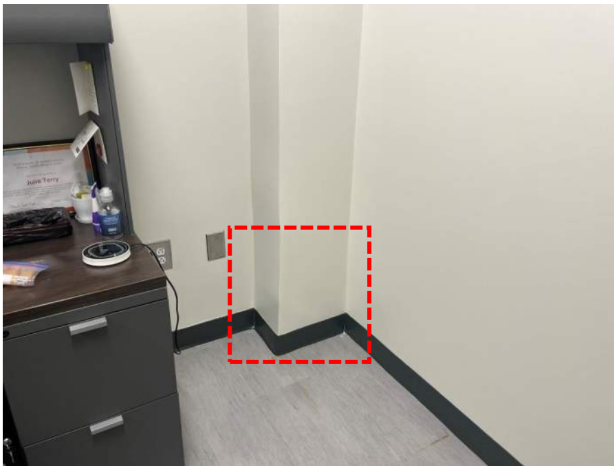
Figure 20. Approximate location of previous interior water leakage reported at southeast corner of Office P108.
