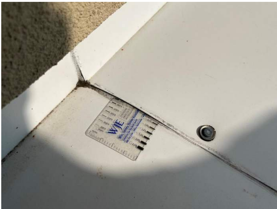
Figure 72. Open gap at the flashing joint.
