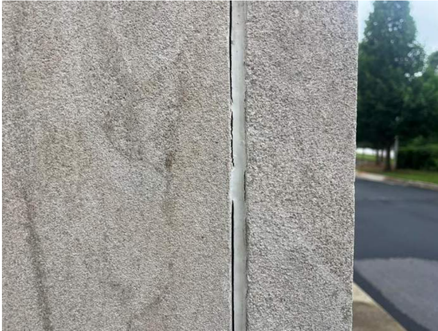
Figure 57. Adhesively failed sealant at limestone panel joint.
