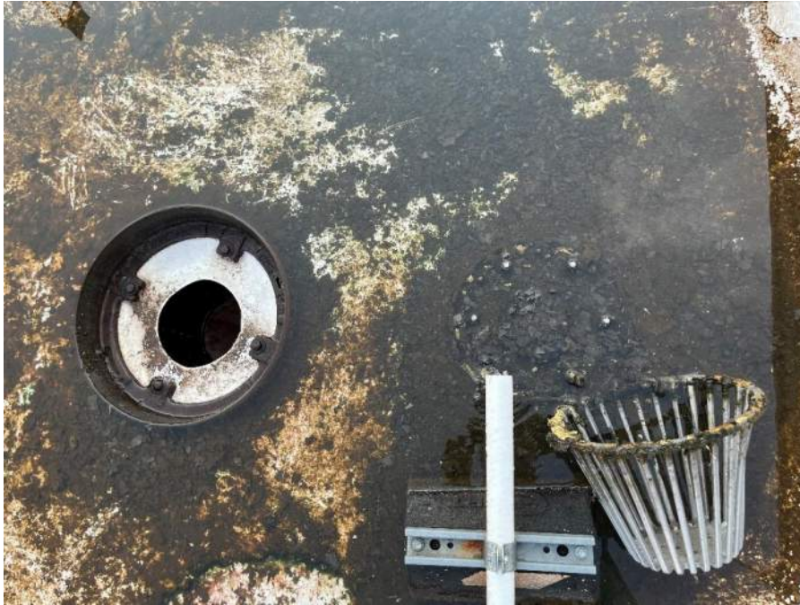
Figure 95. Ponding water at the western half of the main roof and east low roof was concentrated around obstructed roof drains
