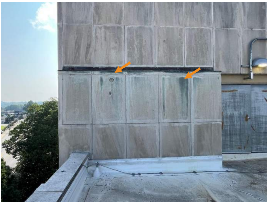
Figure 54. Panels stained green below copper flashing at facade of mechanical penthouse.
