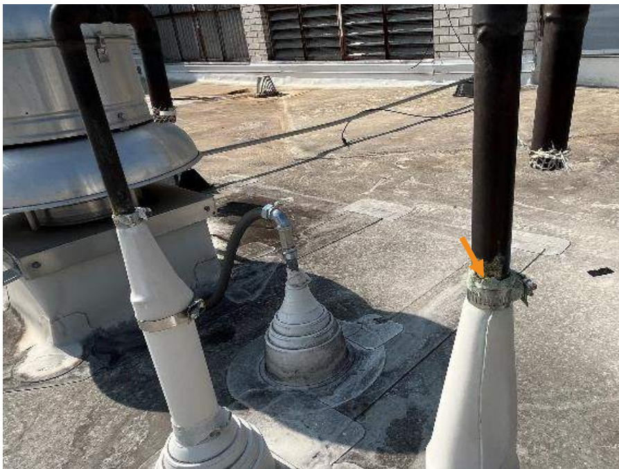
Figure 106. Sealant adhesively failed at copper pipes
