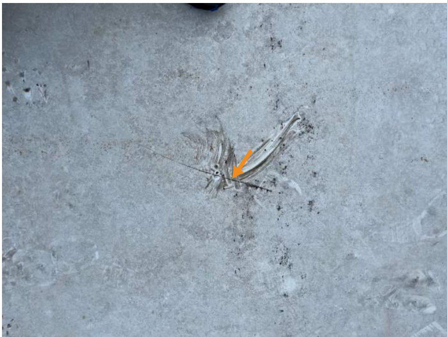
Figure 100. Punches and scratches on the roof membrane
