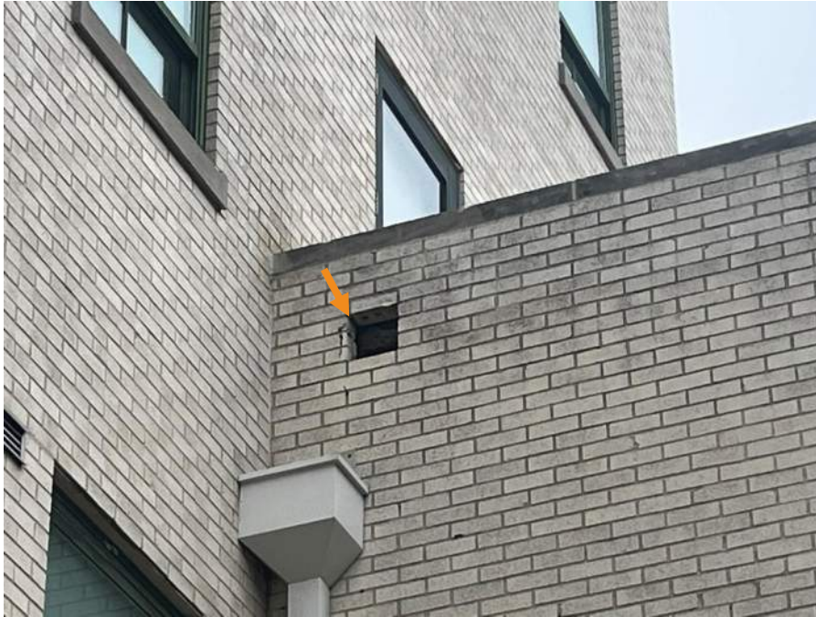
Figure 37. Opening in brick at base of low roof parapet wall.
