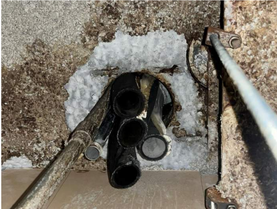
Figure 19. Water staining surrounding a pipe sleeve with numerous abandoned conduits
