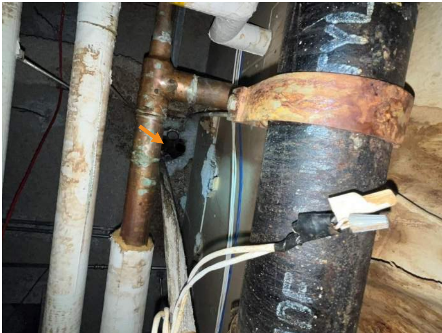
Figure 18. Pipe sleeve (orange arrow) and water staining at concealed roof space.
