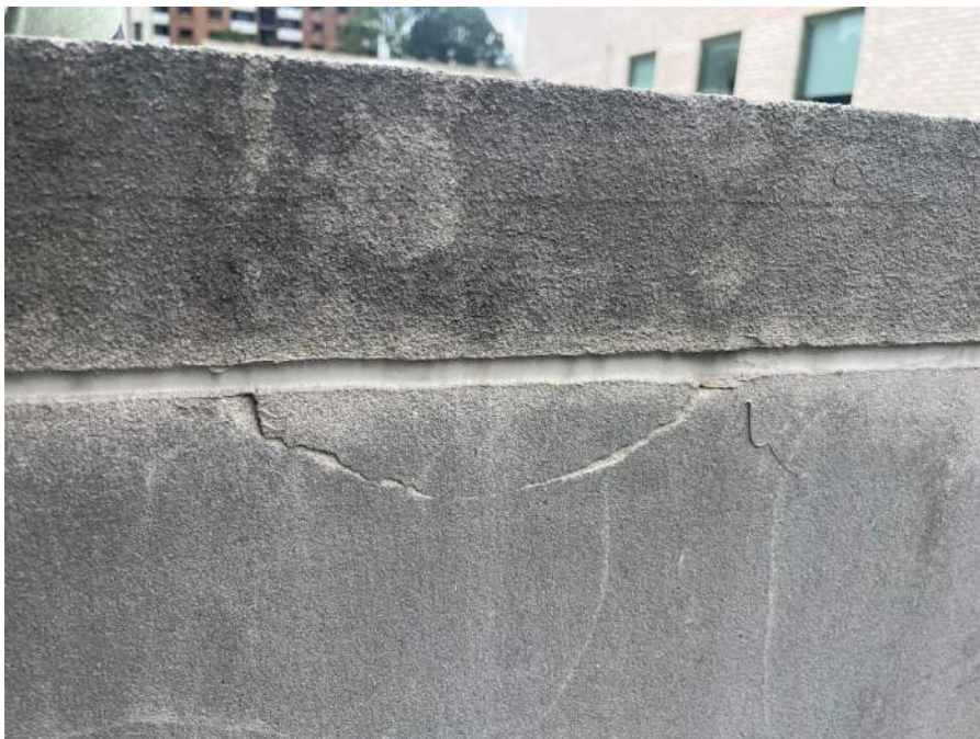
Figure 44. Half-moon cracking below the low roof coping.
