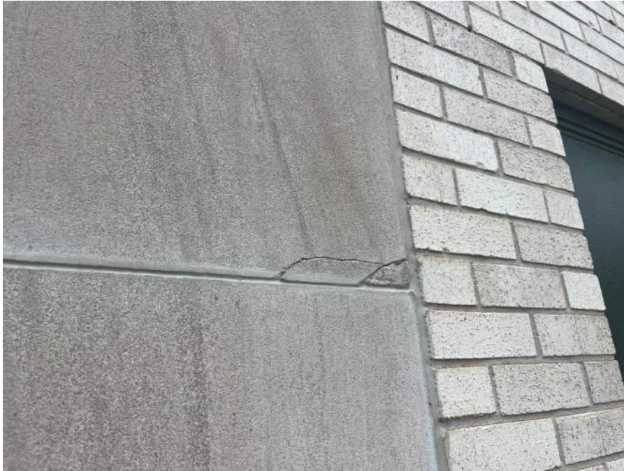
Figure 43. Typical half-moon cracking at panel corners.
