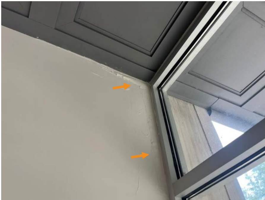
Figure 10. Bubbled and peeling interior finishes adjacent to storefront assembly at north building entrance.
