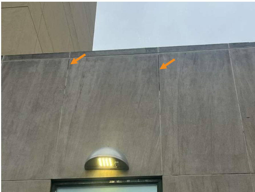
Figure 58. Missing sealant at limestone panel joints.
