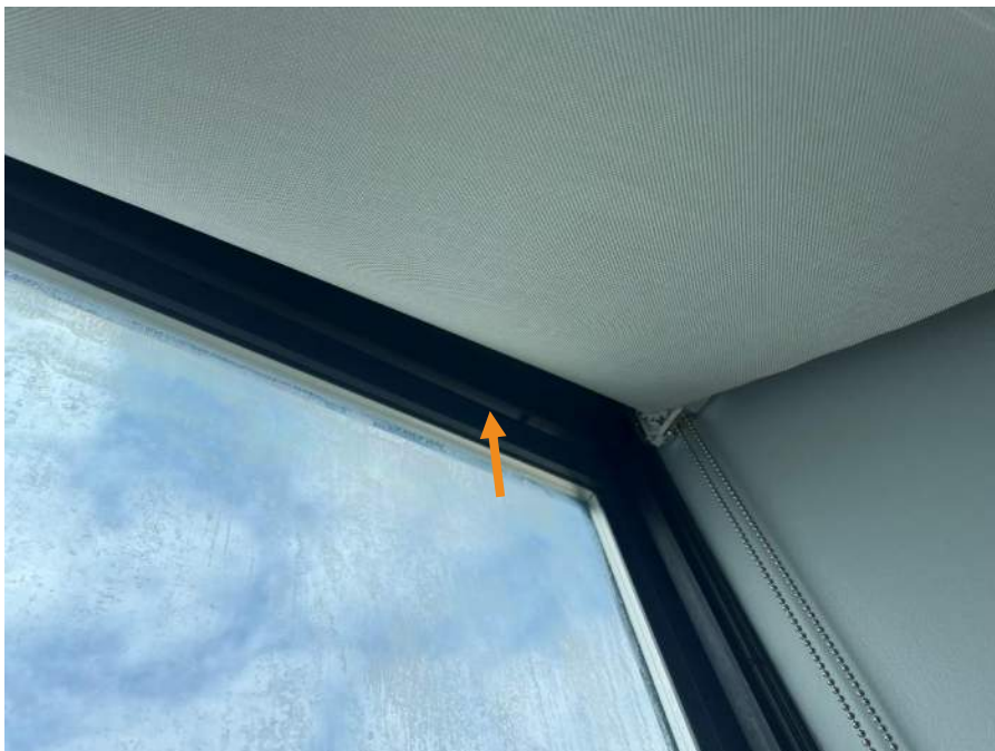
Figure 16. Visible daylight at window upper sash in Group Room 6041
