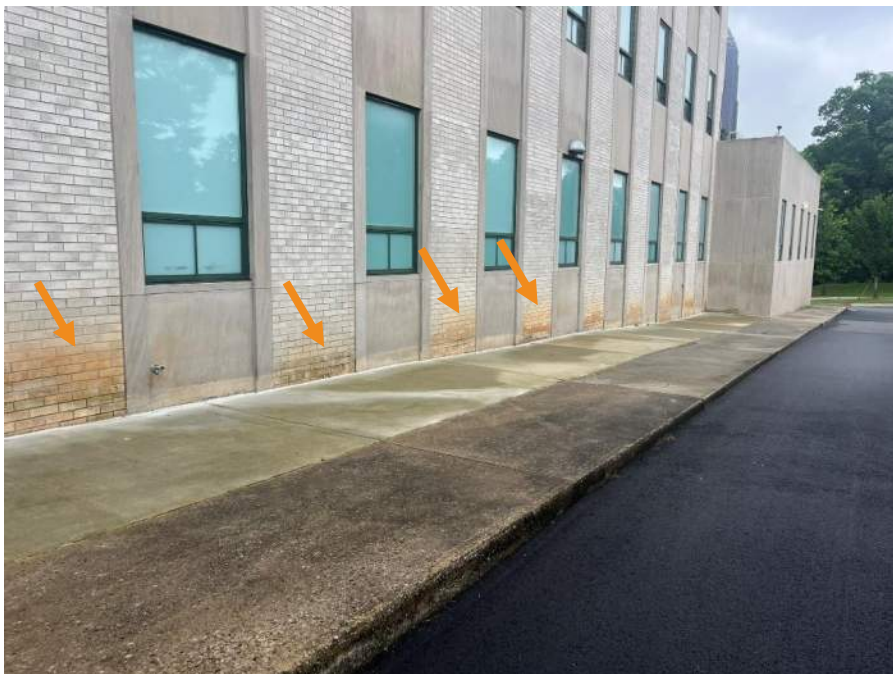
Figure 32. Areas of stained brick masonry at lowest 2 feet along north facade.
