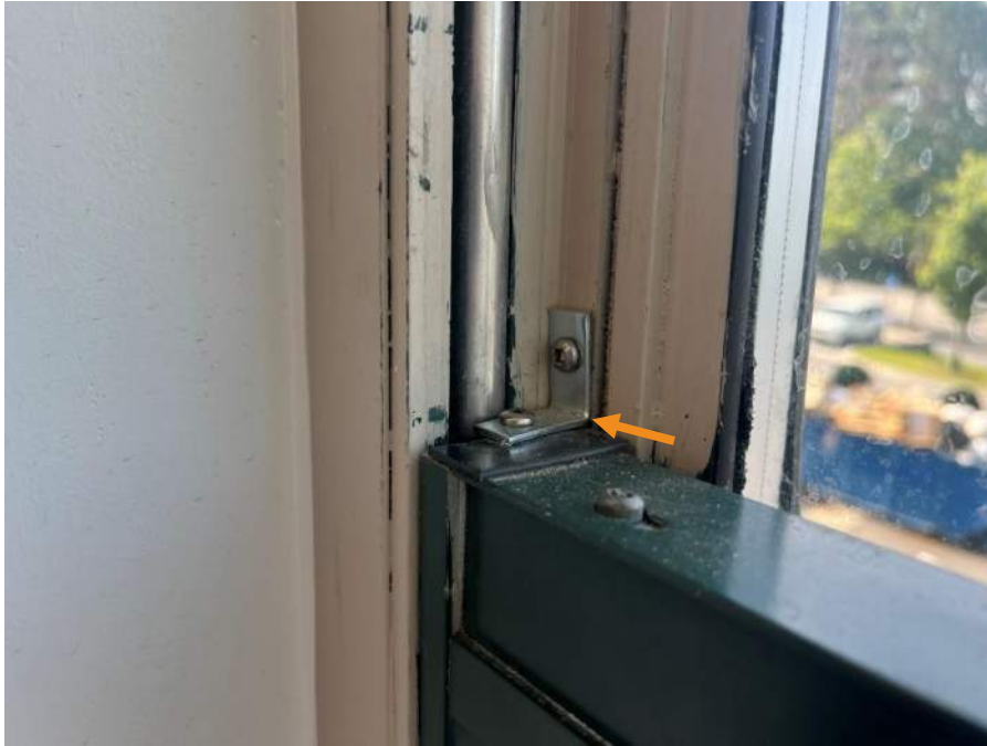
Figure 15. Window unit fastened shut.
