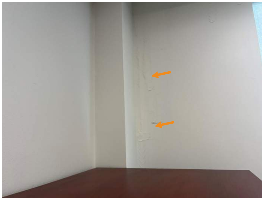
Figure 8. Close-up view of peeling interior finished in Office 6022
