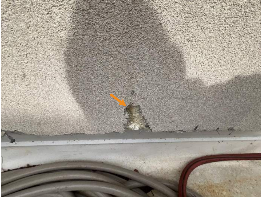
Figure 71. Isolated impact damage exposing the insulation board and mesh.
