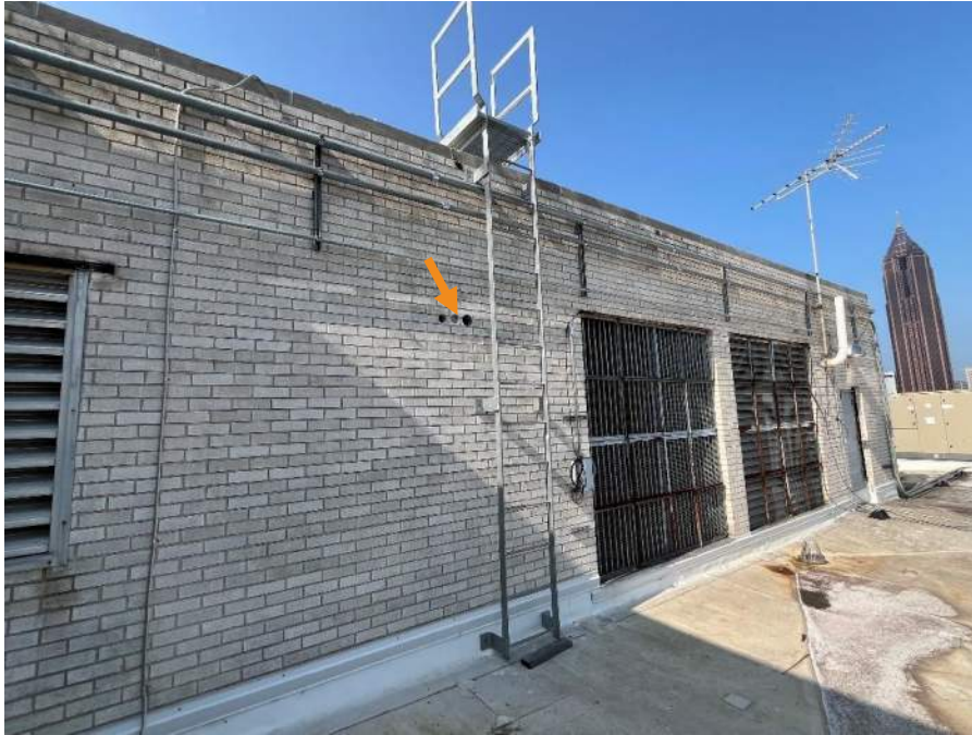
Figure 39. Abandoned penetrations through brick units at the north facade, viewed from the main roof.
