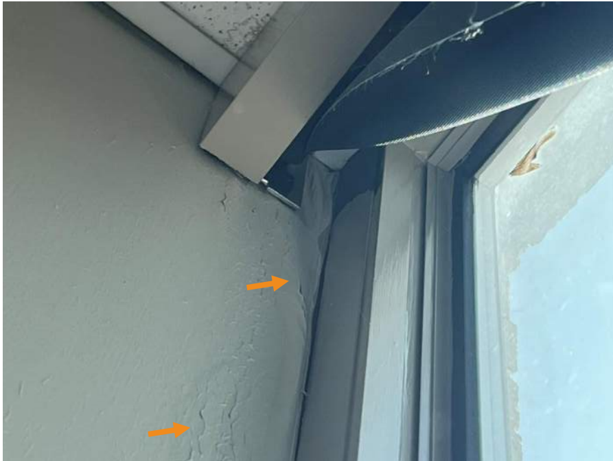
Figure 5. Separated and peeling interior finishes adjacent to window.
