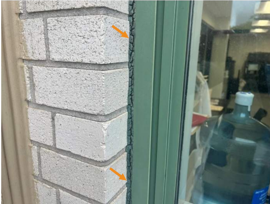
Figure 83. Crazed window perimeter sealant.
