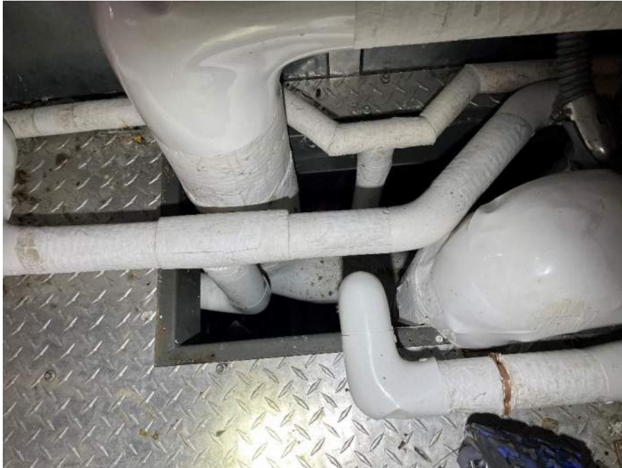
Figure 111. Mechanical and plumbing lines extending into the interstitial space between the mechanical system and roof below
