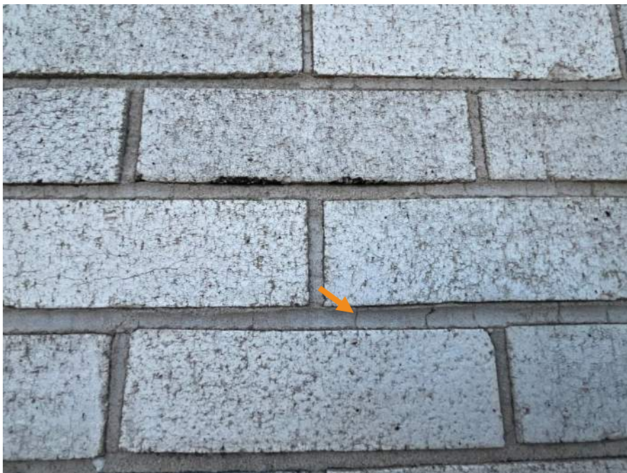
Figure 28. Transverse cracks in mortar joints.
