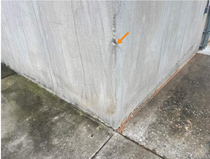
Figure 47. Panel cracking at northwest outside building corner
