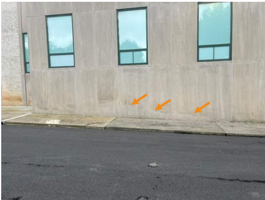
Figure 56. Panels discolored along base of facade at panels extending below grade level.
