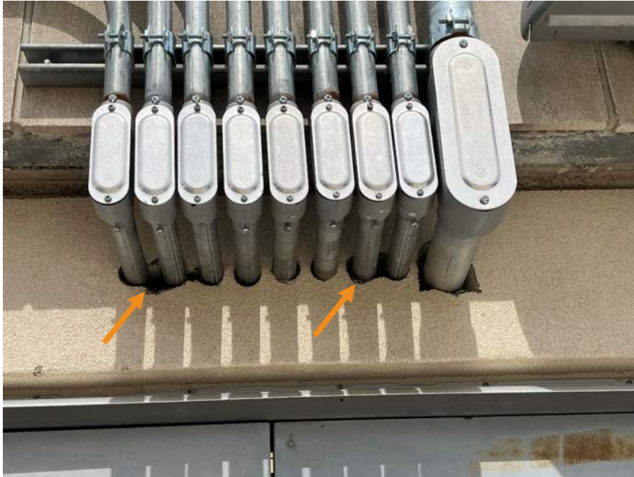
Figure 75. Open and unsealed electrical conduit penetrations through EIFS at the east facade.
