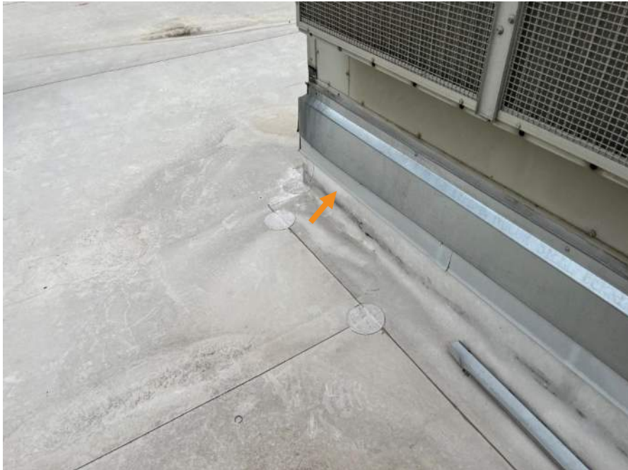
Figure 109. TPO membrane terminated onto mechanical system curb
