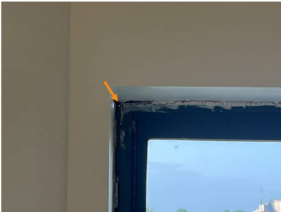
Figure 14. Daylight visible between window head-jamb corner and interior finishes.
