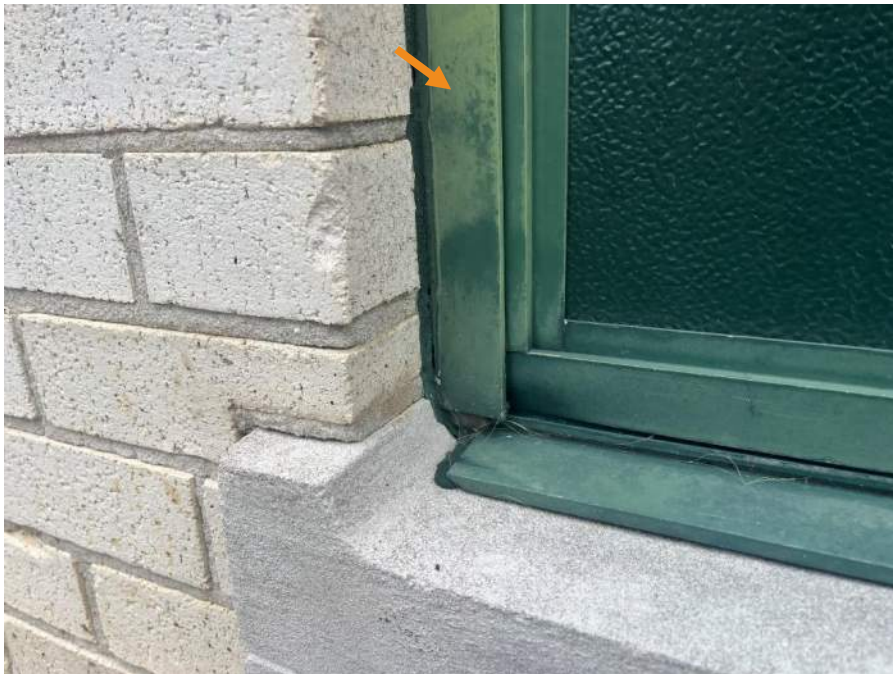
Figure 82. Weathered window frame coating.
