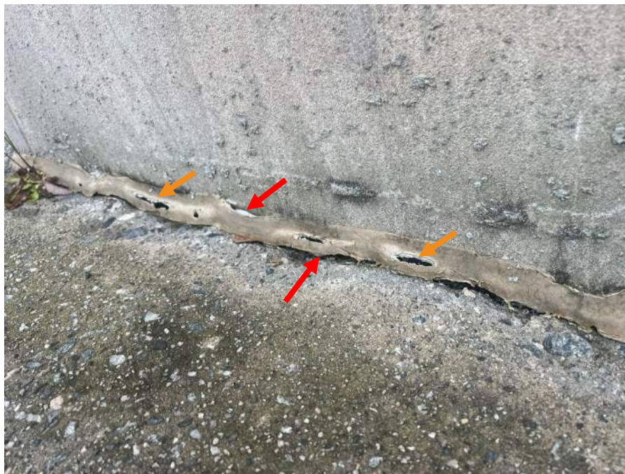
Figure 60. Close-up view of adhesive (red arrows) and cohesive (orange arrows) failure of sealant installed between limestone panels and grade.
