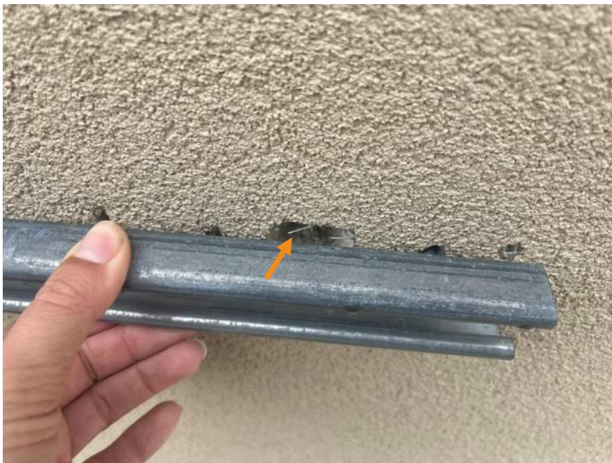
Figure 74. Abandoned Unistrut channel concealing exposed EIFS mesh and insulation.
