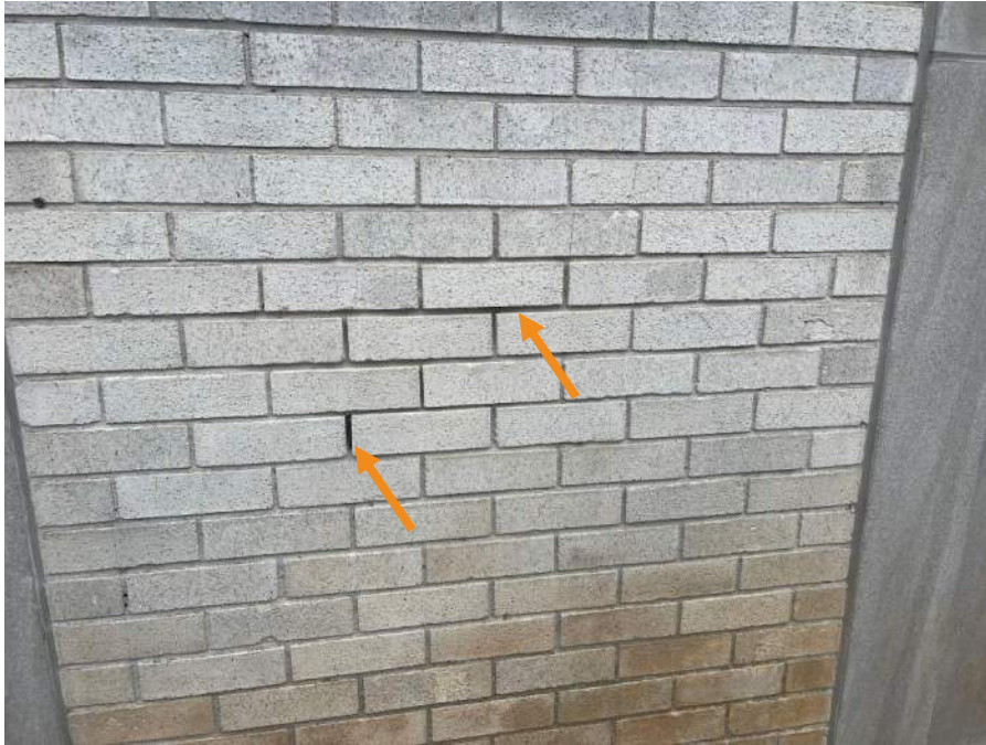
Figure 31. Area of eroded mortar and stained brick masonry.
