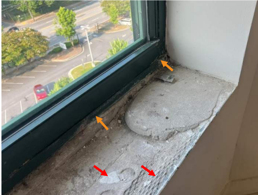
Figure 13. Staining along base of window frame (orange arrows) exposing metal lath extending from plaster finishes and inside surface of the brick backup wall (red arrows)
