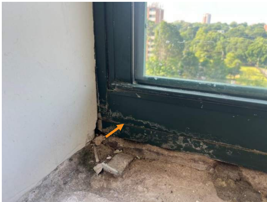
Figure 4. White staining at window frame joint.
