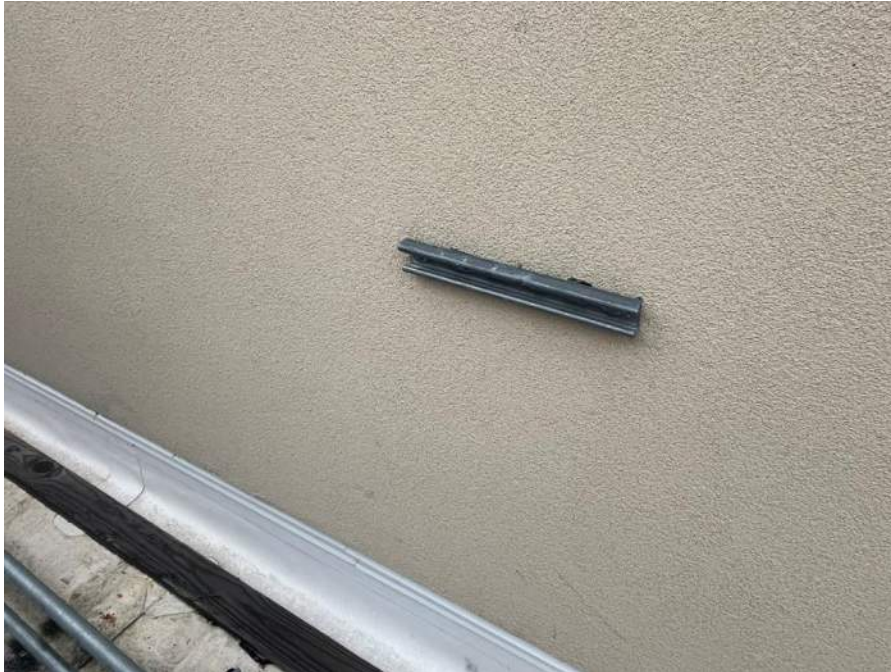
Figure 73. Abandoned Unistrut channel at the west wing low roof.
