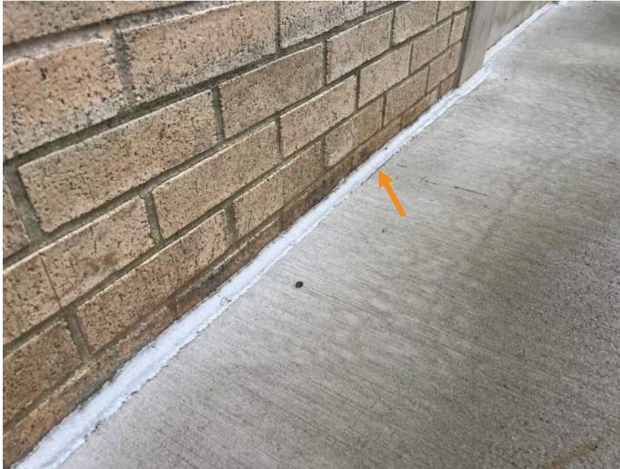
Figure 35. Adhesive failure of sealant installed between brick masonry and grade along north facade.
