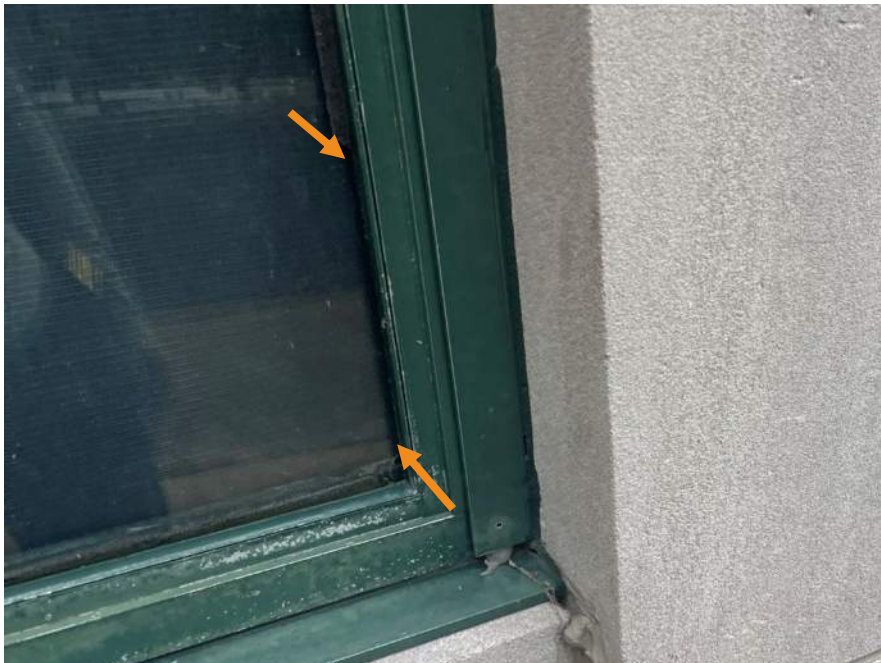
Figure 88. Missing portion of glazing gasket at north facade ground floor unit
